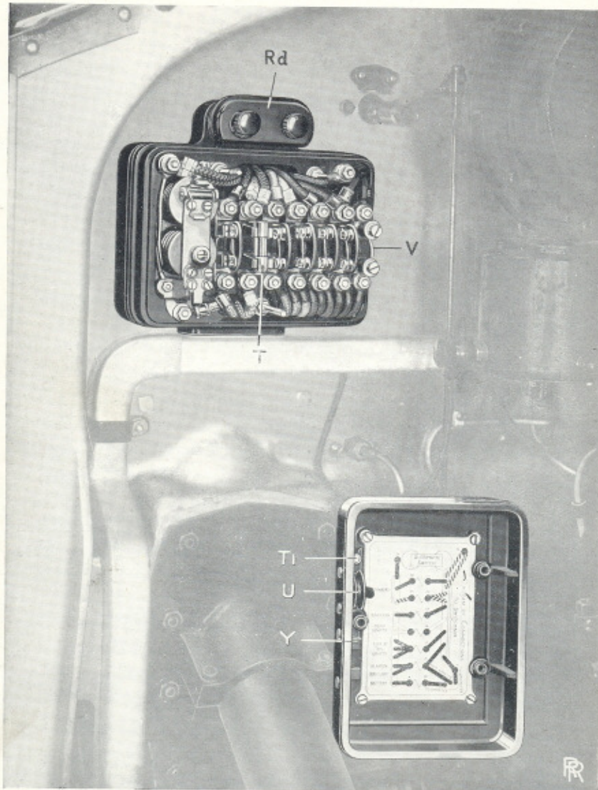
FIG. 33. DISTRIBUTION BOX, WITH COVER REMOVED, AND DYNAMO FIELD RESISTANCE.
